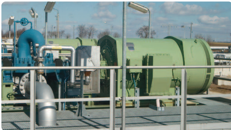
Pump drives in a pipeline booster station Powered by a Schorch, Ex de IIB T4, 1450kW, 6kV, 2 pole motor
